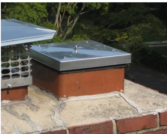
Top mounted damper for fireplace.
