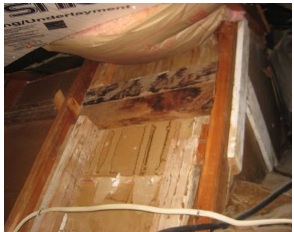
Old water stains.
