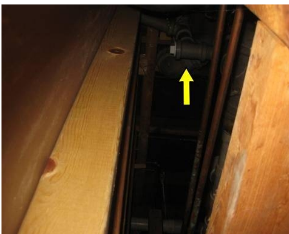
Galvanized waste pipe.
