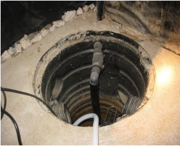
Pump for french drain system.
