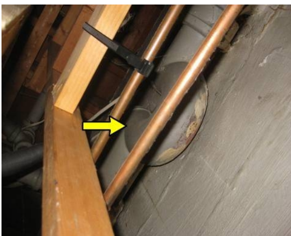
Behind laundry room wall.
