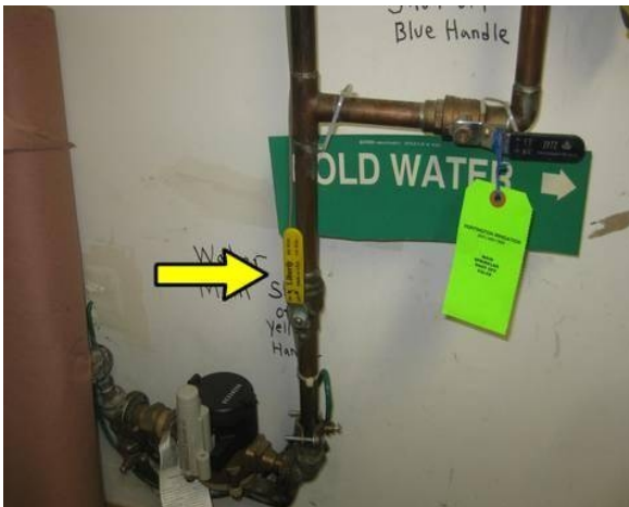
Main water shutoff.
