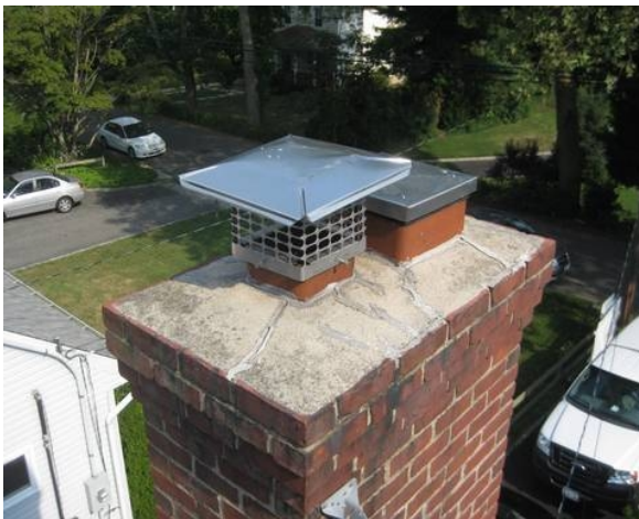
Seal cracks better.
