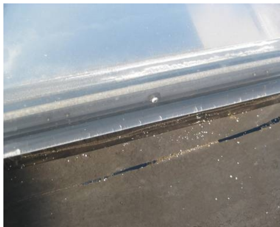
Outer covering starting to crack.
