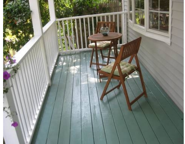
Deck looked ok.
